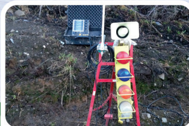
GAS MONITOR SYSTEM W/ ALARM
